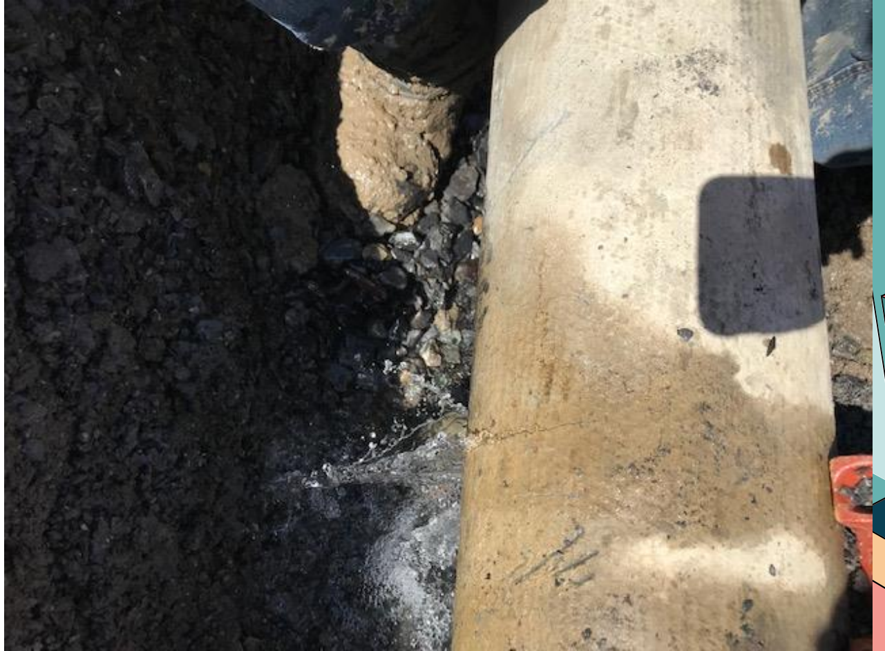
Cracked asbestos-cement pipe
