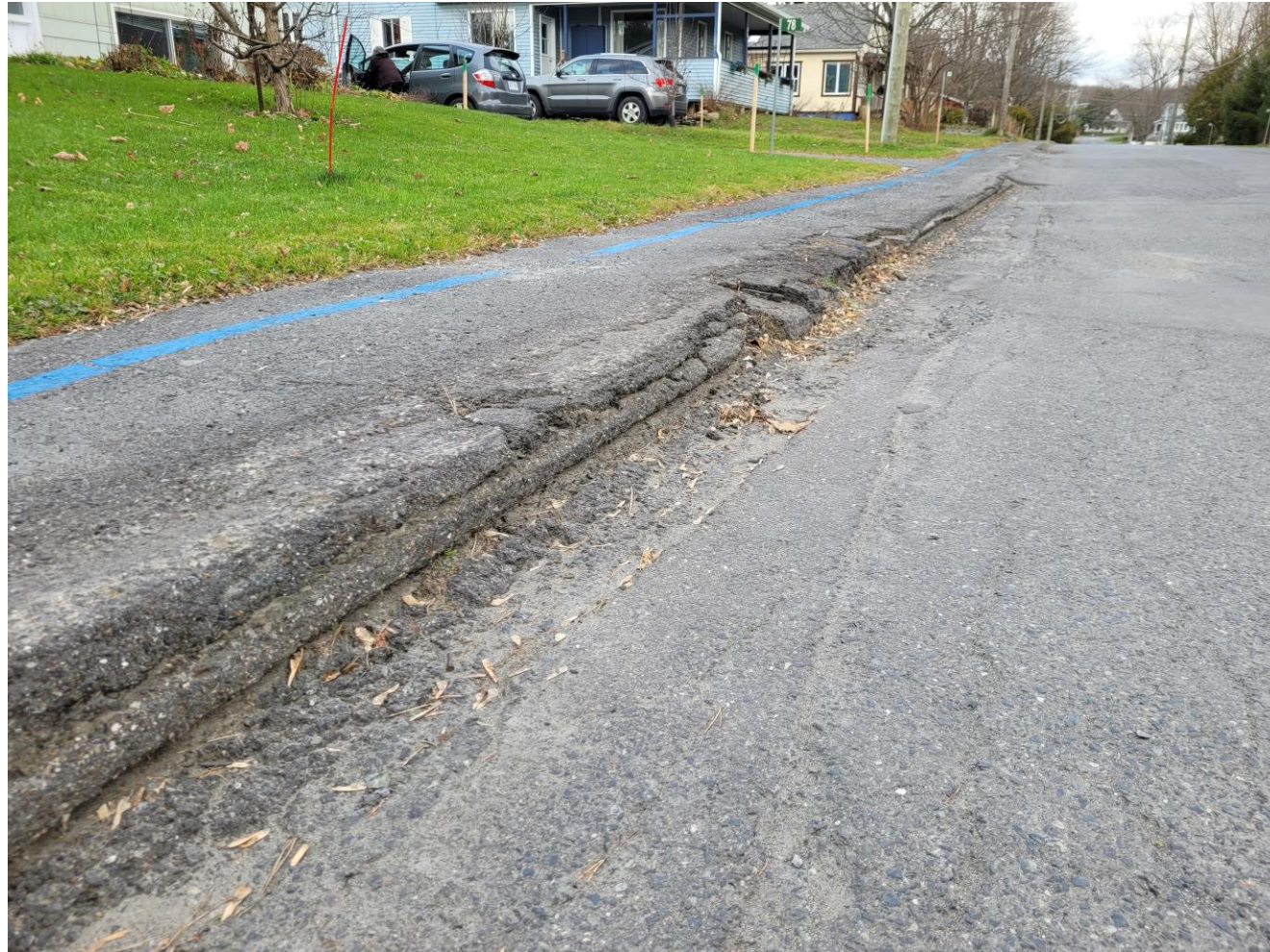
Asphalt sidewalks, degraded and dangerous
