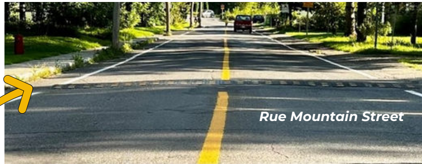
Installation de dos d'ânes temporaires sur les rues Western et Mountain Installation of temporary speed bumps on Western street and Mountain street
