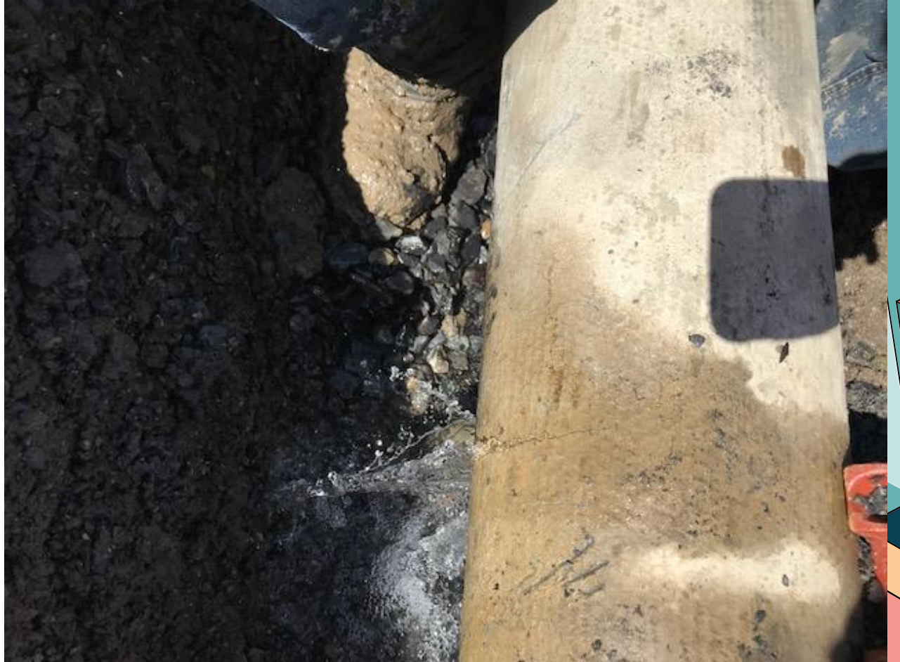
Cracked asbestos-cement pipe
